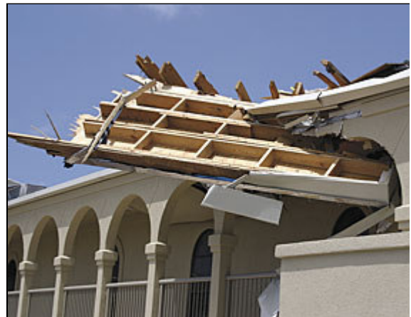
A portion of the sanctuary roof ripped off Our Lady of the Assumption Church crushed the roof of Hunt Hall, the parish hall at the mission church on Pensacola Beach.
